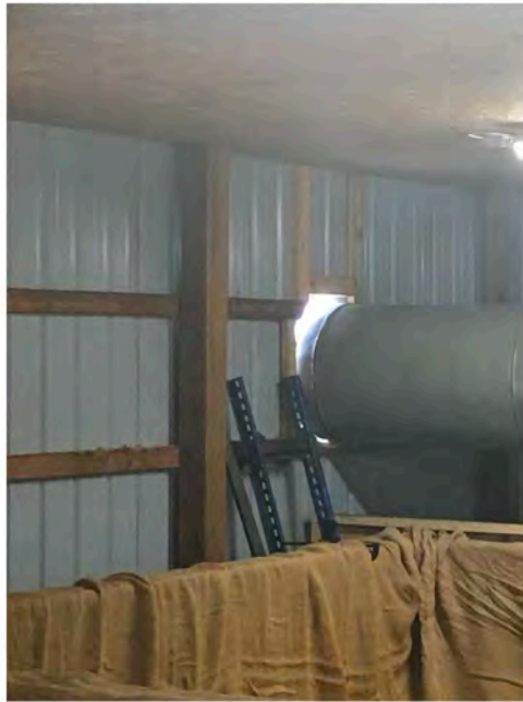
Sealing these cracks would be great.
